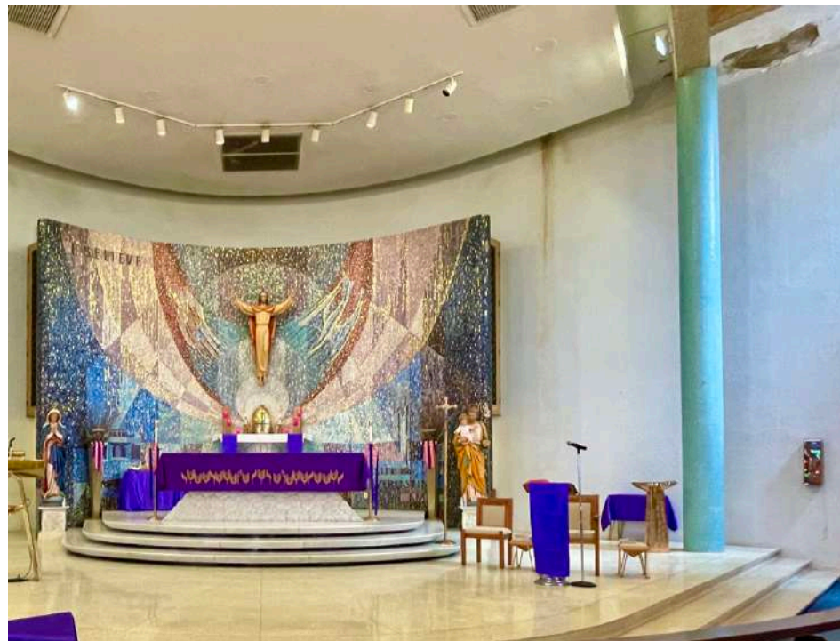
With the roof failing, plaster ceilings have begun to spall and break apart (upper right corner). Ceramic tiles are also beginning to fail.
