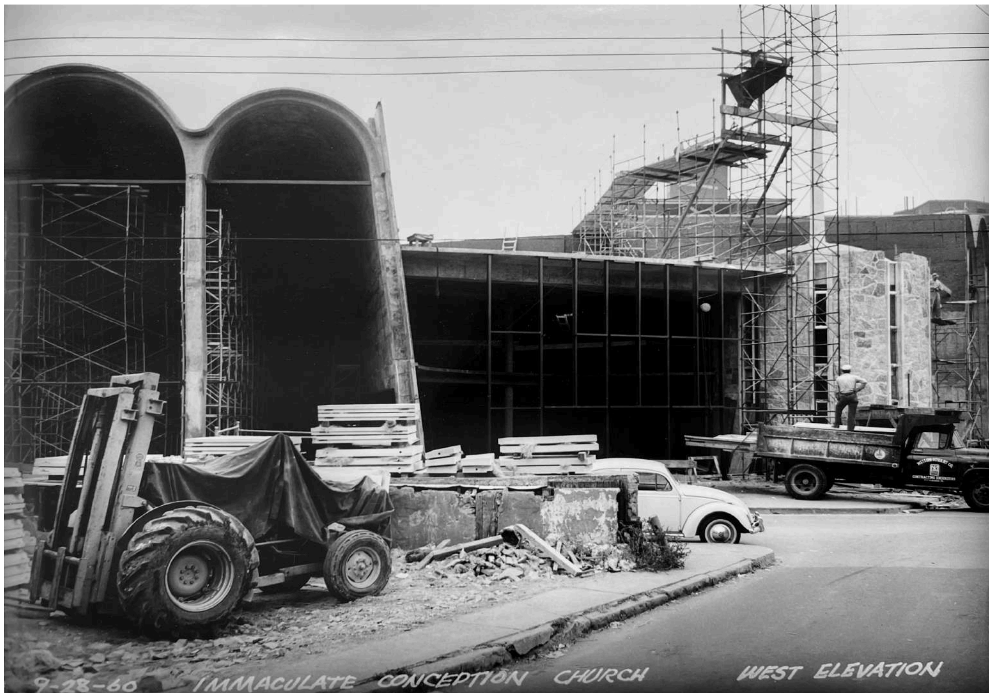
West Nave and Narthex, September 28, 1960. Scaffolding and formwork are removed to reveal the cavernous space of the west nave and narthex.
