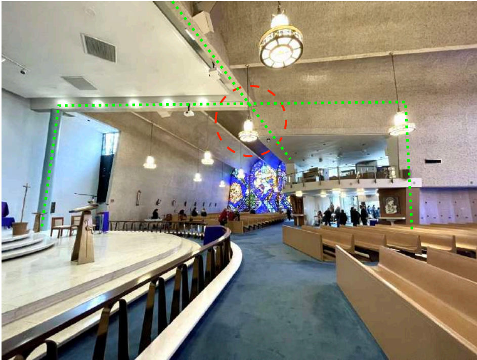
Barrel vaults of the south and west naves are supported by two immense beams at about 80' in length (dashed in green).
