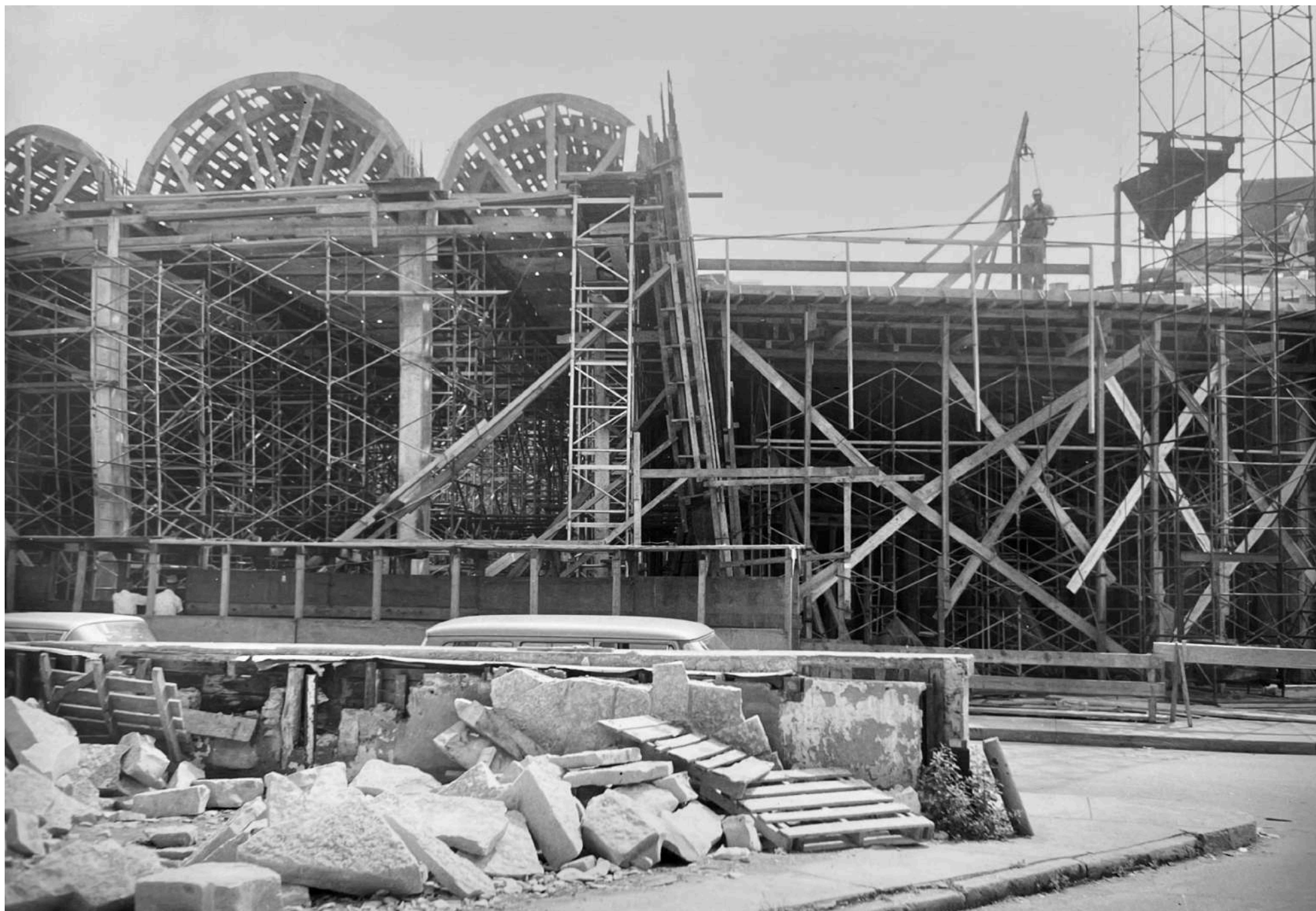
West Nave and Narthex, July 27, 1960. In the foreground, the first house on the block opposite the church is demolished, opening the view to the new church.
