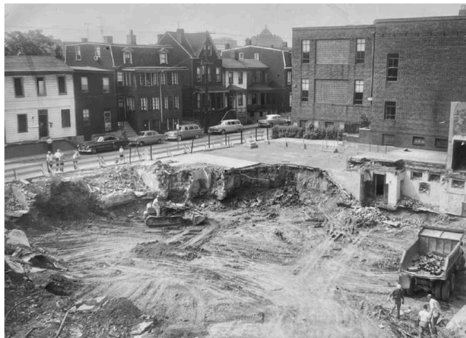
Site work began on August 3, 1959 with the demolition of the old church.
