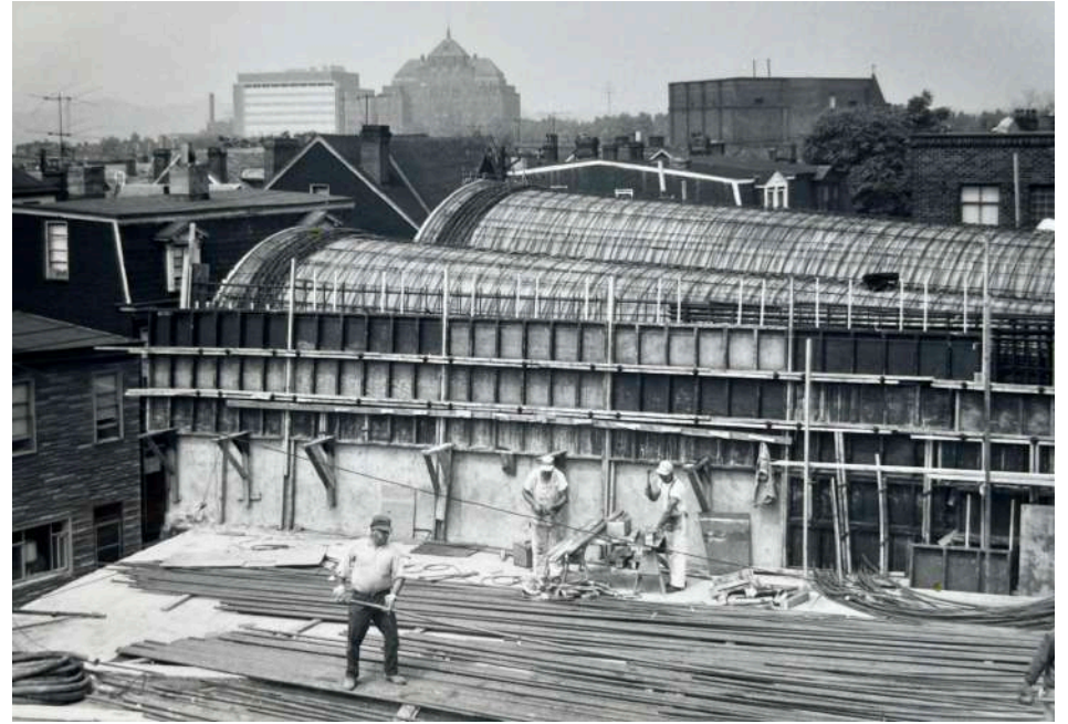
The walls of the church were cast first before the roof formwork was installed.
